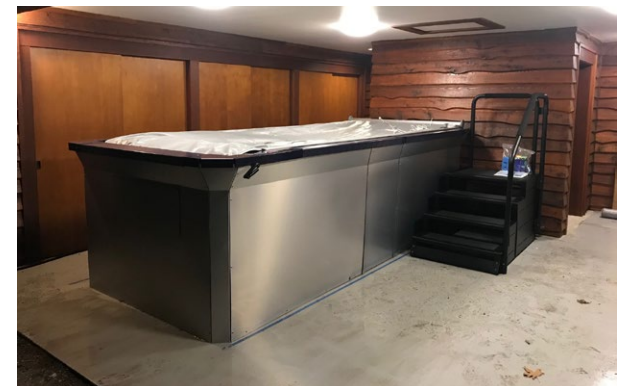
Aboveground Indoor Installation
